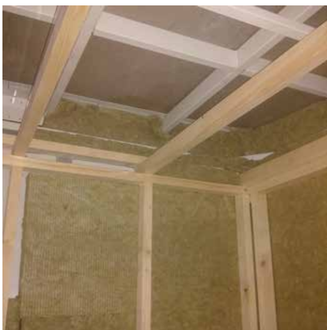
Showing first layer of insulation prior to the rolled insulation being fitted
